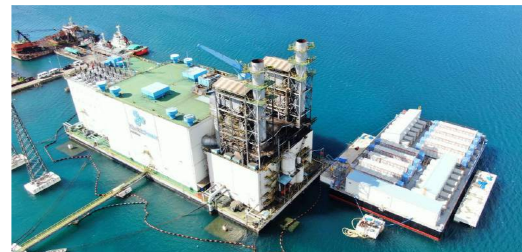
As the country’s economy grows, so does the need for power. AboitizPower’s Therma Marine facility in Maco, Davao de Oro is the site of the company’s latest BESS project.
